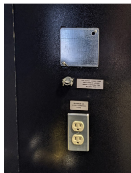
Electrical Supply Junction Box
