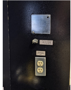
Electrical Supply Junction Box
