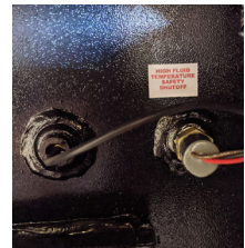
High Temp Safety Shutoff
