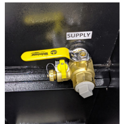
Supply Valve (closed)
