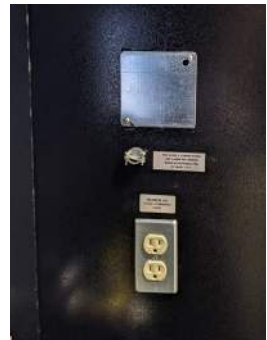
Electrical Supply Junction Box
