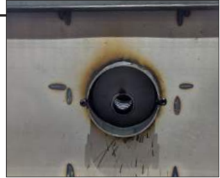
Combustion Air Tube
