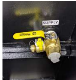
Supply Valve (closed)
