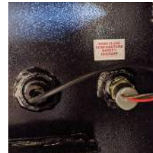
High Temp Safety Shutoff
