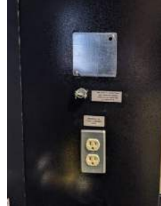
Electrical Supply Junction Box
