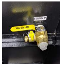
Supply Valve (closed)
