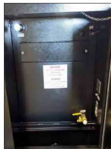
Rear of Furnace
