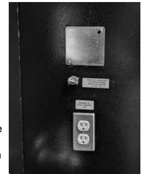
Electrical Supply Junction Box
