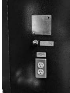
Electrical Supply Junction Box
