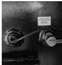
High Temp Safety Shutoff
