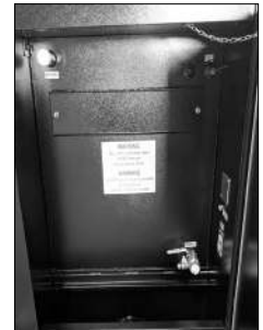
Rear of Furnace
