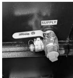
Supply Valve (closed)
