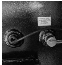
High Temp Safety Shutoff
