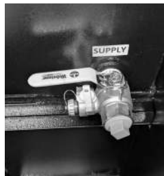
Supply Valve (closed)
