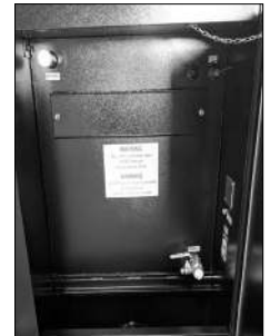
Rear of Furnace
