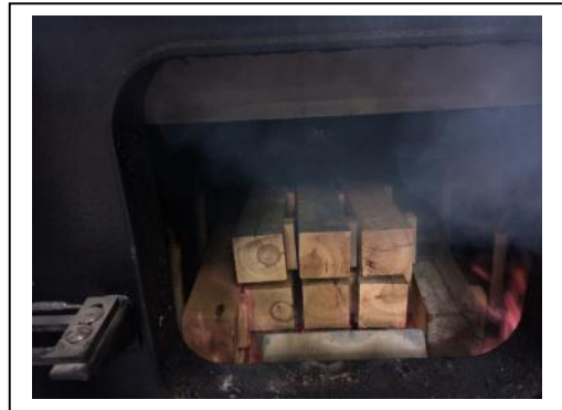
Run 7 J Newly Loaded Boiler
