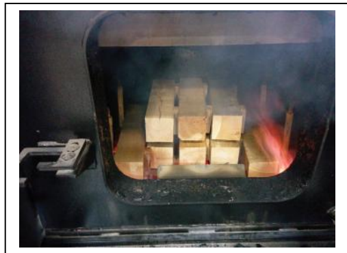
Run 6 J Newly Loaded Boiler
