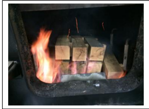
Run 2 J Newly Loaded Boiler
