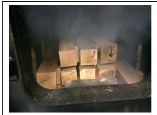
Run 3 J Newly Loaded Boiler
