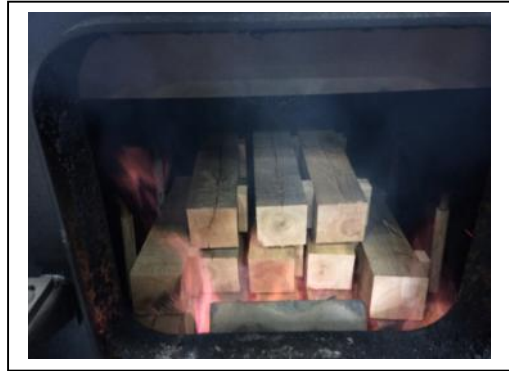
Run 5 J Newly Loaded Boiler
